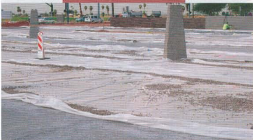
Recently poured concrete is covered with plastic and carefully sealed during the curing process.
