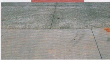
Sidewalks are built using conventional concrete and elevated slightly to drain onto the pervious concrete.
