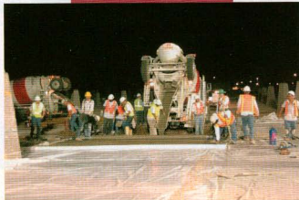
Night shots showing the pouring of the 3.4-acre park-and-ride lot being built of pervious concrete at Glendale Avenue and Loop 101 in Glendale, Ariz. Three photos courtesy Stew Waller
